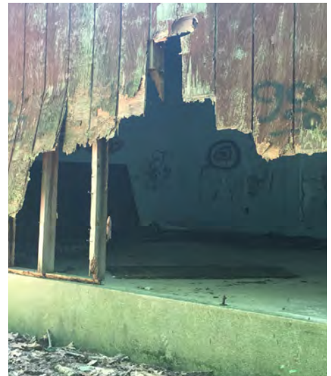
Run down building (Image 3.2.8.2)
