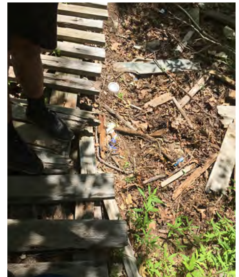
A half-broken wooden bridge (Image 3.3.3.3)
