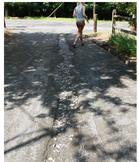
Erosion on driveway (Image 3.6.5.5)
